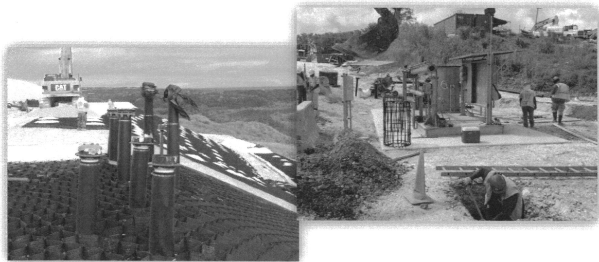
Figure 11 Gas collection system components (Gas extraction wells and Gas Flare)
