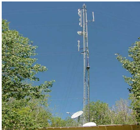
Image 2: Sample picture of a telecommunication antenna site.
