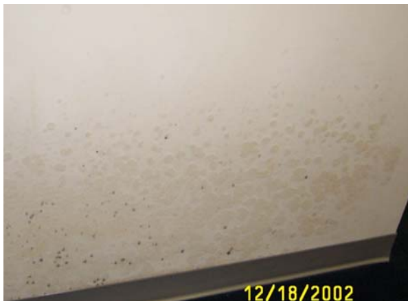
Mold grew all over the walls at the OPA after Supertyphoon Pongsona caused major water damage to the building.
